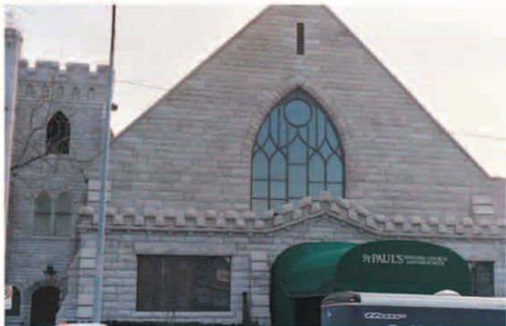
This 5/8-in. plate-glass protective glazing system was installed in a new mahogany wood frame at St. Paul's Episcopal Church in Kansas City, MO.
